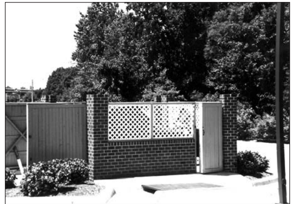
Dumpsters and other unattractive features and areas should be screened from public view by attractive methods such as this masonry and lattice fence.
